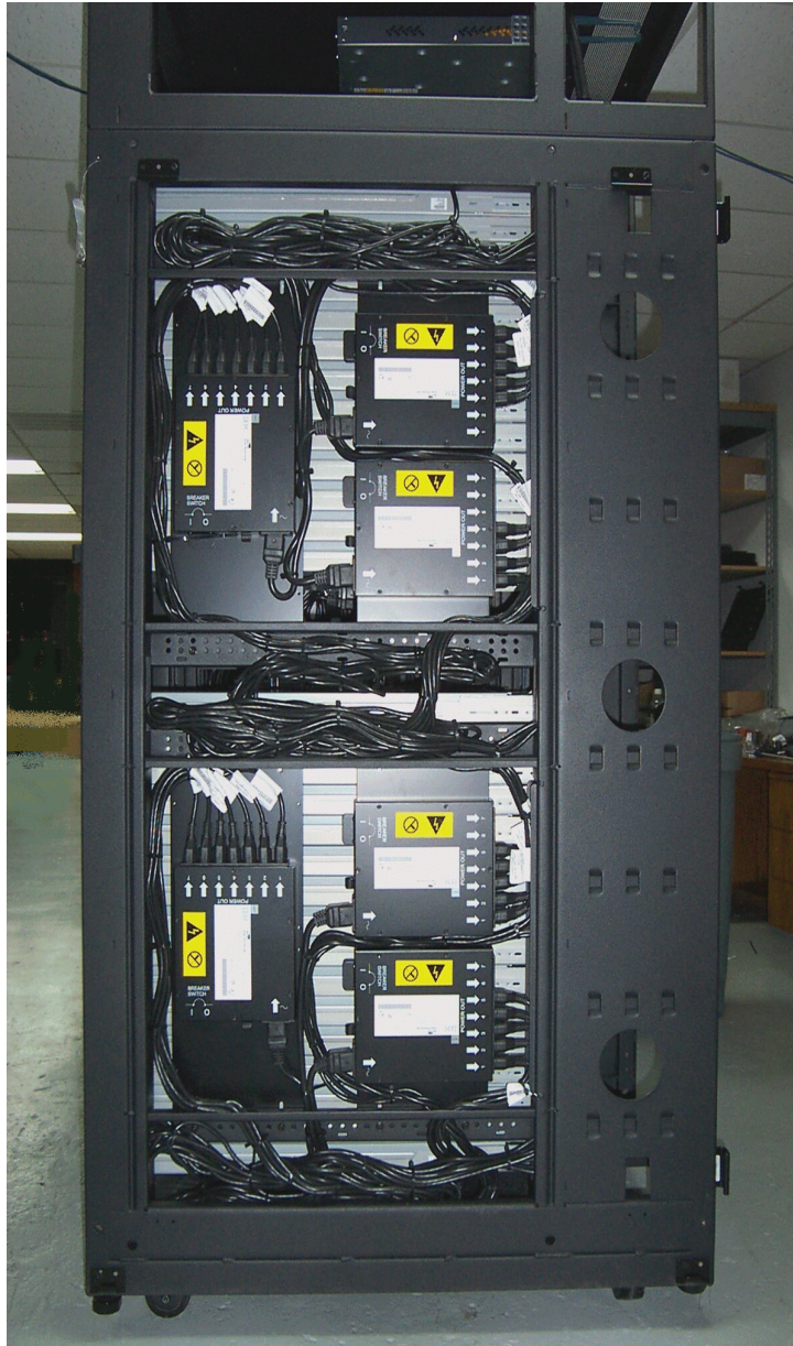
Figure 3-4 Power distribution units
